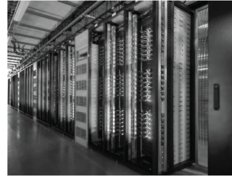
Data Center Services
